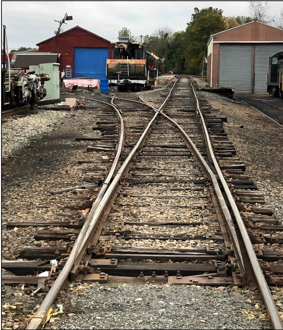
View of Black River & Western main track facing North at Ringoes Switch No. 7. Approximately 282' of existing track, including the turnout shall be removed and replaced with CWR.
