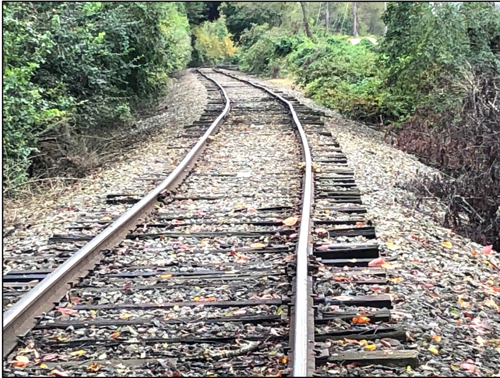
View of Black River & Western main track facing South through the 'S' curve at Milepost 7.5+/- . Existing track shall be removed and replaced with 132#RE rail on steel and composite ties.
